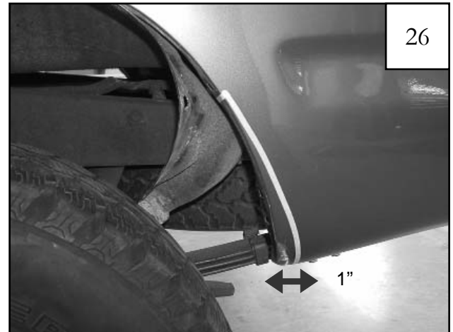
Measure out 1" at bottom of rocker. Make a tape line from bottom of rocker up, intersecting the first tape line. Using a reciprocating saw, cut fender on the inner edge of tape line.
